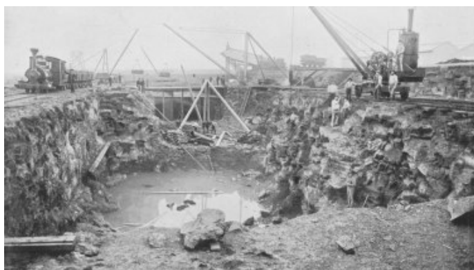
A remarkable undertaking: building a vast sewer and stormwater network by hand and steam-power. Source: Melbourne Water
